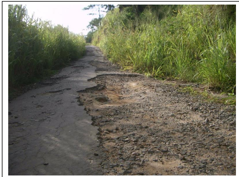
Road rehabilitated by the project in need of maintenance
