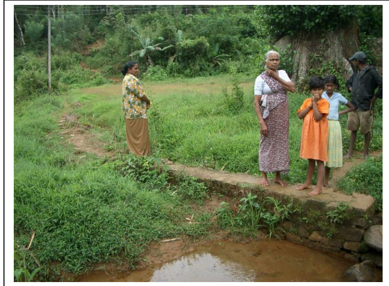
Anicut Rehabilitated by the project in a state of disrepair, Ganga Ihala Korale
